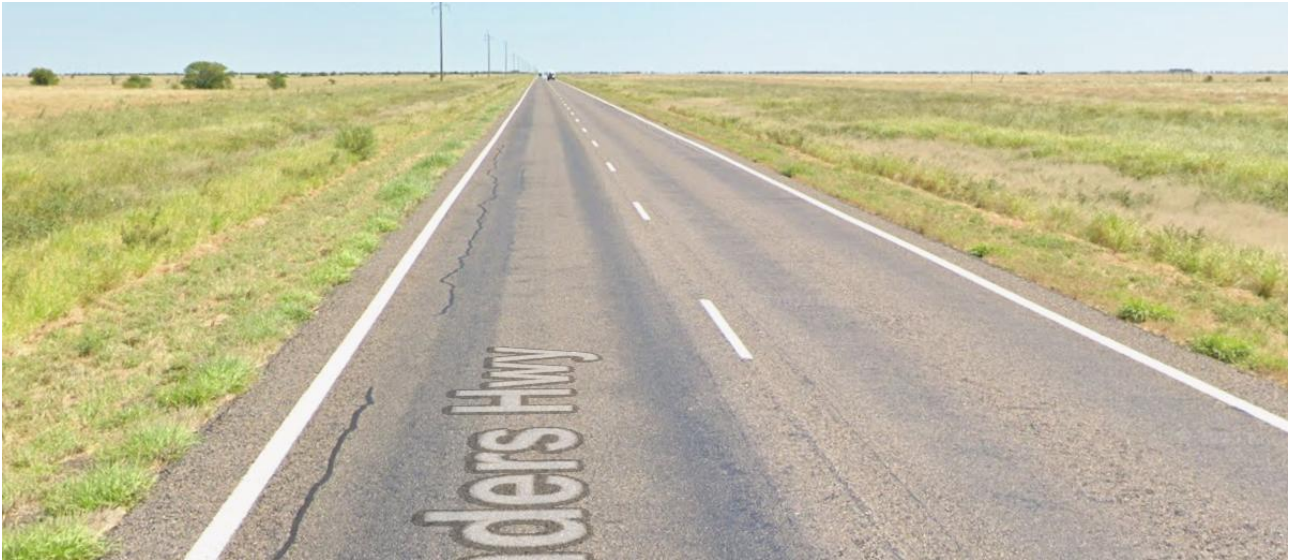
Figure 23: Flinders Highway looking west between Richmond and Julia Creek (Google Maps, April 2023)
